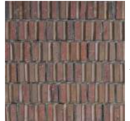
Breno FK6 broken with 2 gaps 120 x 85 mm
